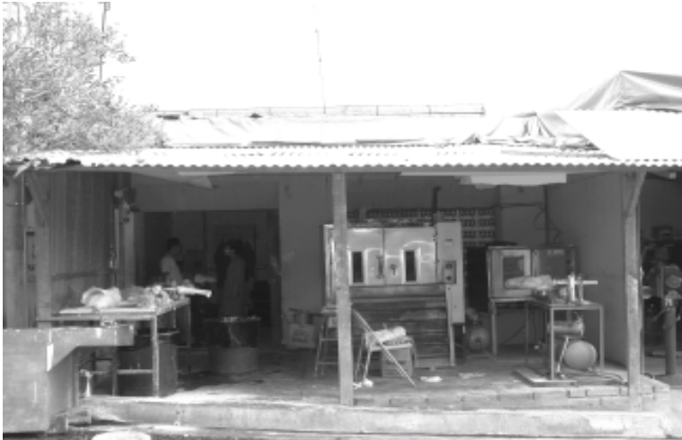
A January 2001 earthquake damaged the main FUNTER building. This was the temporary work shop.
